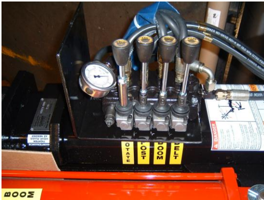
Fig. 3-1 Hydraulic Controls Mounted on Center Post
